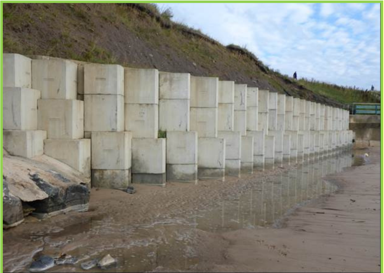
New T-Block units (constructed in 2014) prevent outflanking at the southern end of Trinity Road seawall (/4501C04)
