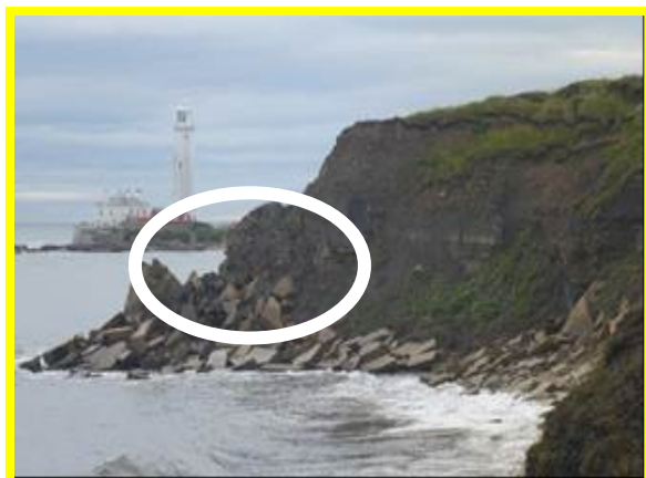
Slippages in soft material along upper cliffs and rock fall at base (/4401C24)
