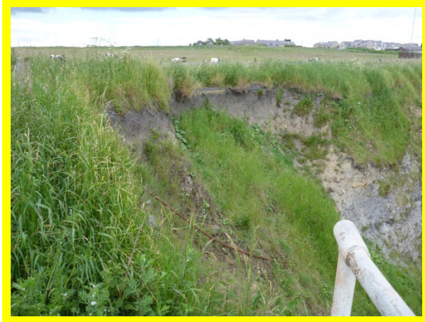
Slippages in soft material adjacent to Hartley Cove access steps (/4401C23)
