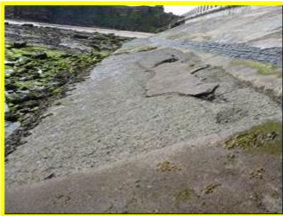
Sea wall in fair condition with abrasion of the apron leading to exposed rebar (/4701C27)
