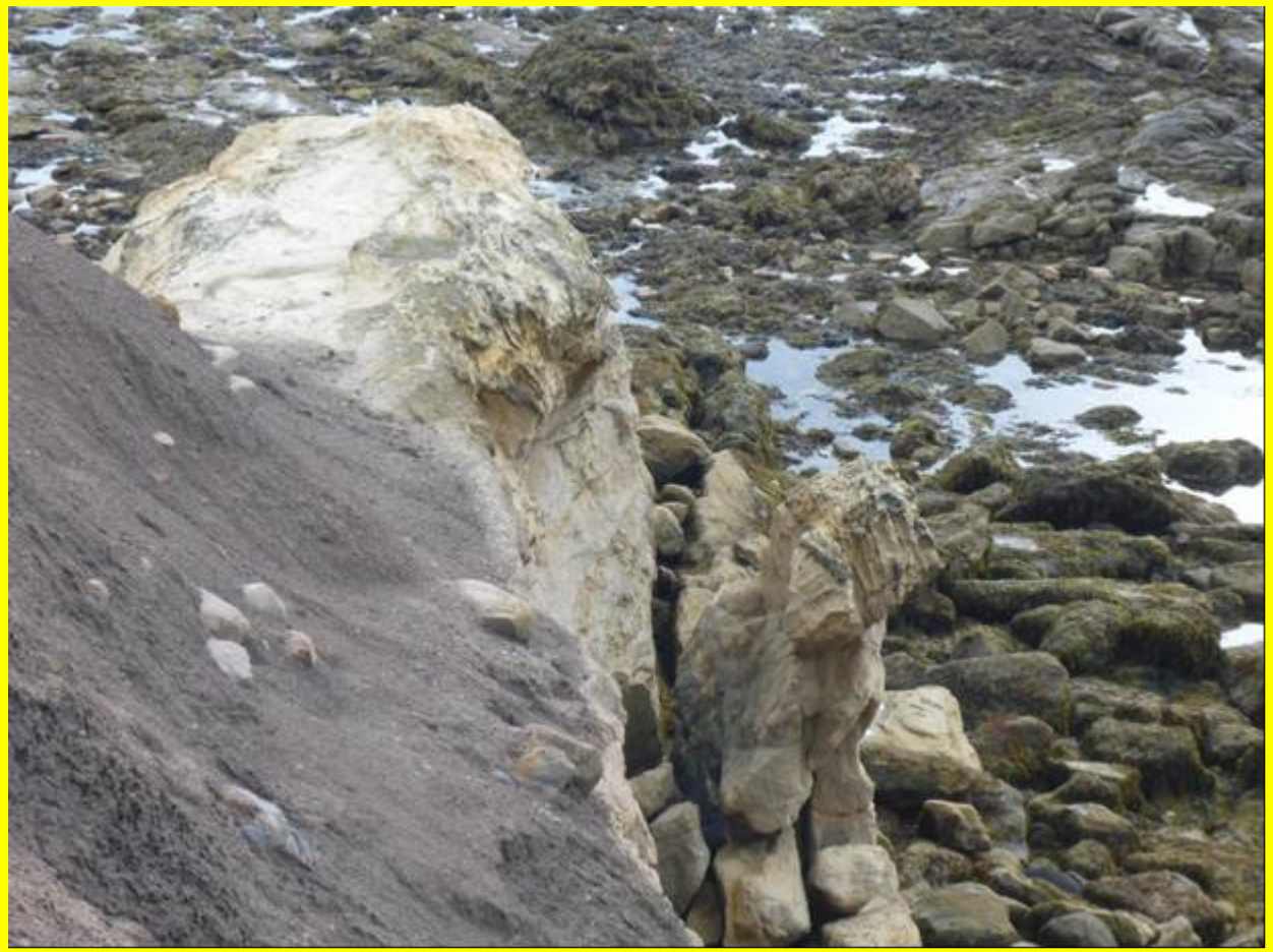
Rock stack near Tynemouth North Point that has the potential to topple imminently (/4701C16)
