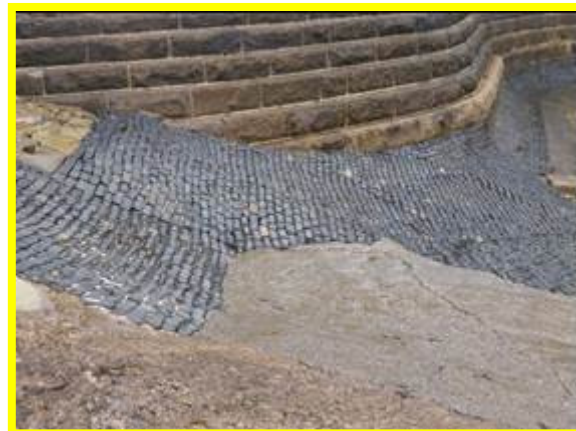
Final section of sea wall in generally fair condition, but with some defects at the tie-in requiring remedial attention (/4701C06)
