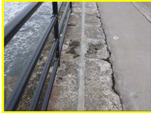
Gaps in promenade deck at northern end (/4601C10)
