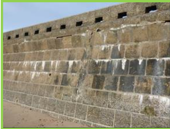
Previous repairs and local open joints which would benefit from maintenance (/4501C07)
