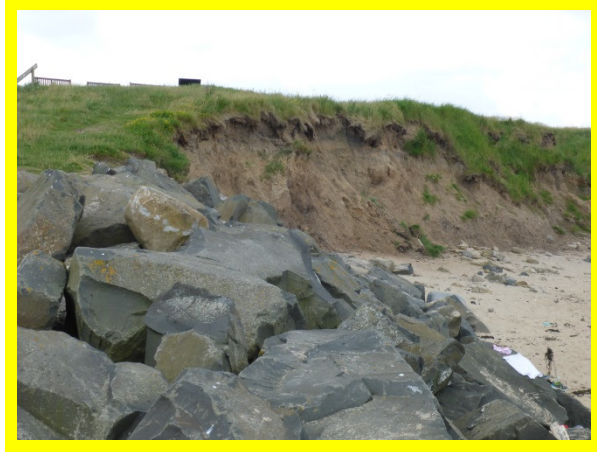
Erosion adjacent to rock revetment by St Mary's Island causeway (/4401C24)
