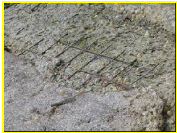
Exposed rebar (/4701C27)
