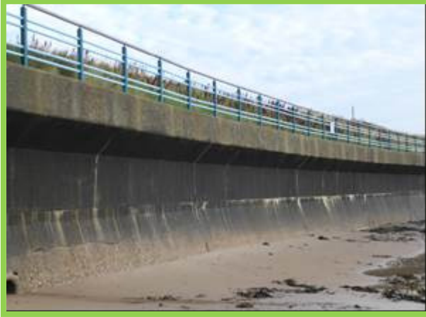
Trinity Road seawall in good overall condition, but with some minor maintenance required (/4501C04)
