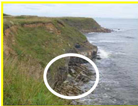
Rock falls in hard material along lower cliffs (/4401C24)
