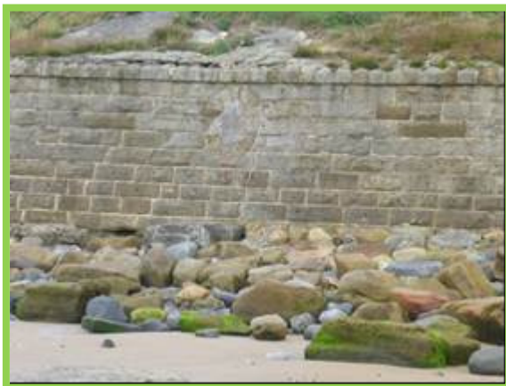
Slumping in cliffs near northern end of masonry wall (/4701C17)
