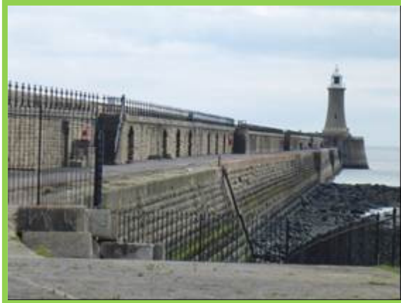
North Pier appears in good overall condition and is well maintained (/4801C01)
