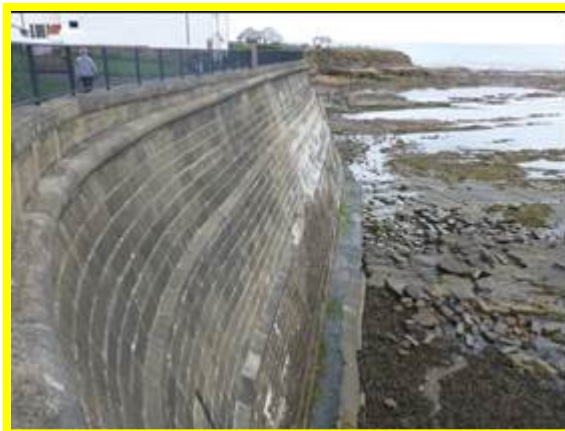
Final section of sea wall in generally fair condition, but with some defects at the toe requiring remedial attention (/4701C06)
