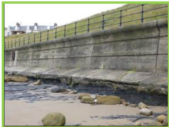
Undercutting and exposure of coal at toe of wall (/4701C18)
