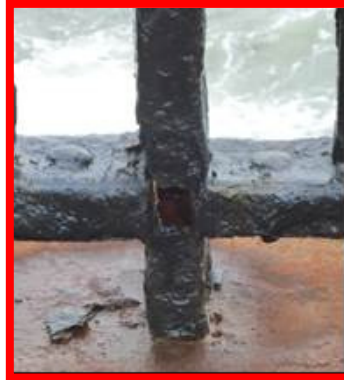
Broken handrailing (/4601C06)
